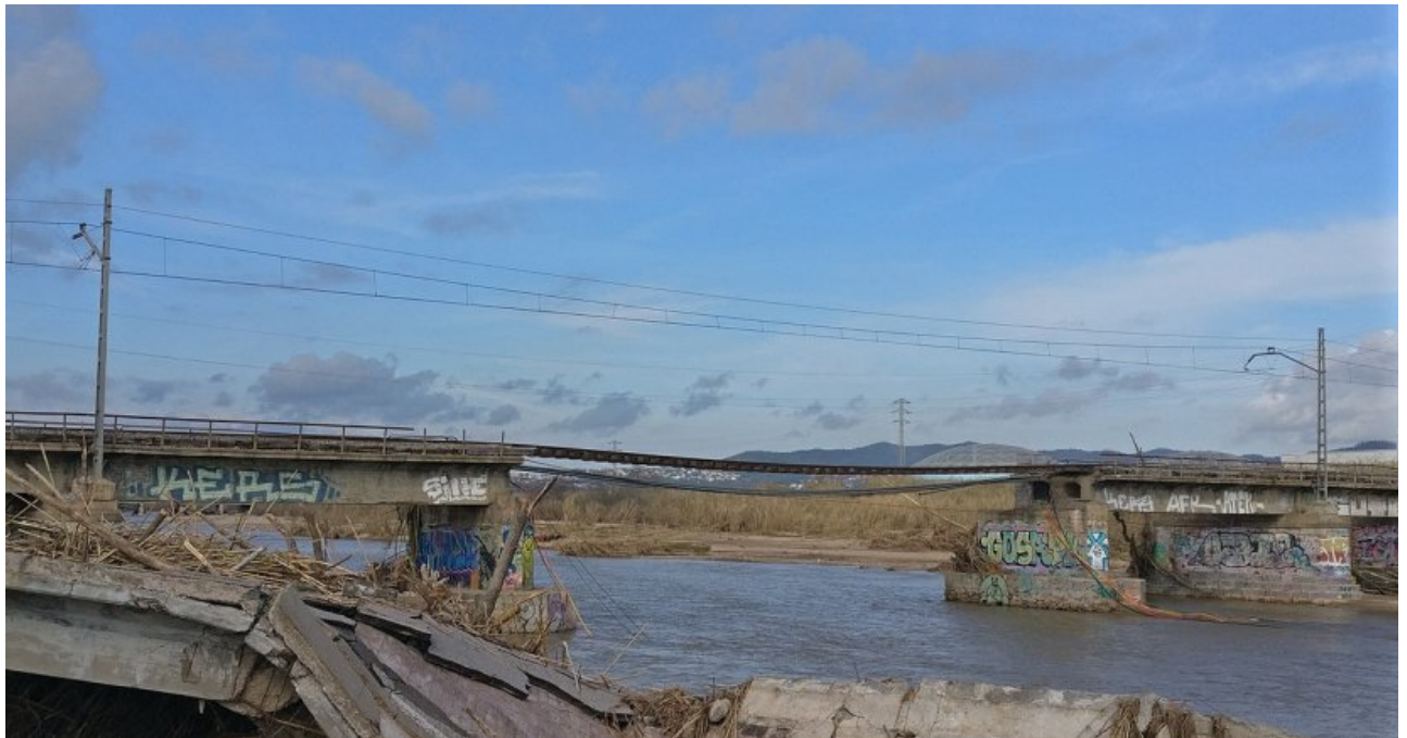
Destruction of the Tordera road and railway bridges during the Gloria storm (January 2020) © Wikipedia
